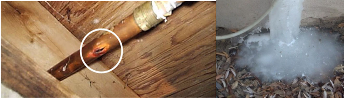
Split pipe inside the house and leakage outside the hose bib
